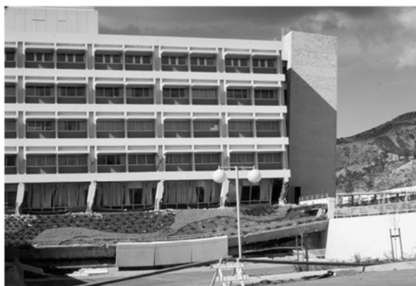
FIGURE 13.5 Permanent offset of weak first story due to discontinued wall, Olive View Hospital, 1971 San Fernando earthquake. (Photograph by K. Steinbrugge, used with permission from the National Information Service for Earthquake Engineering, University of California, Berkeley.)
