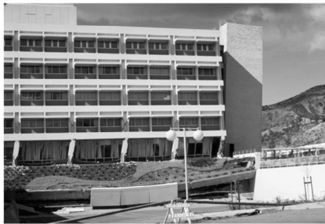
FIGURE 13.5 Permanent offset of weak first story due to discontinued wall, Olive View Hospital, 1971 San Fernando earthquake. (Photograph by K. Steinbrugge, used with permission from the National Information Service for Earthquake Engineering, University of California, Berkeley.)
